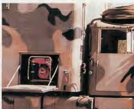
Access to the auxiliary gasoline generator is through a trapdoor on the right side of the van body that used to service the photo lab.
