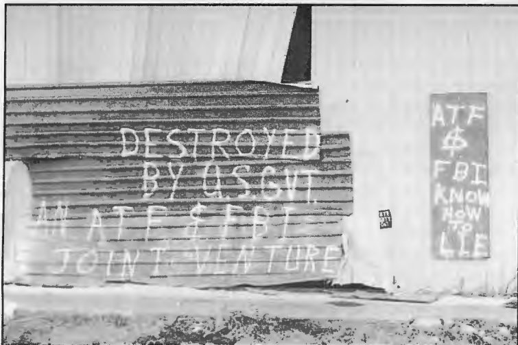
Rented building of Mag Bag, David Koresh's auto repair business, deliberately wrecked by ATF agents in Bradley fighting vehicle. Building's owner, banker Gary Welch, stood by with keys in hand, begging agents not to destroy his property. When he objected, he was arrested. Photo: James L. Pate
