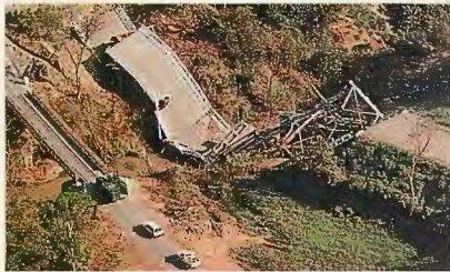
Bridge over Coyolate River on main southern coast road CA2 between Mexico and El Salvador, blown with estimated 200 pounds of TNT during early morning hours of 12 December 1989. ORPA was blamed for blast, but some officers speculate privately that it was a foreign job, evidenced by professionalism of the work.
