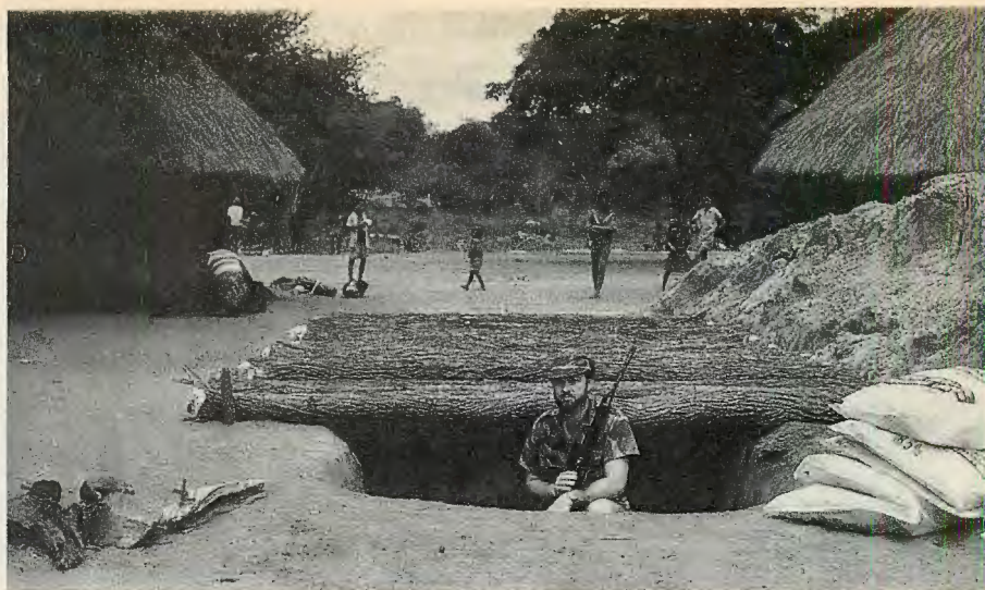
Top: Nearly completed dugout constructed in Tracker Unit residential compound for protection from mortar attacks. Bottom: Final touches are put on the dugout. When finished, structure will protect against all but heaviest direct hits.
